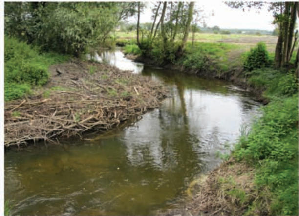
Brush wood berm created using locally won material felled to enable access for machinery.
